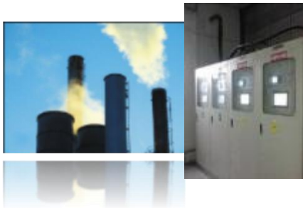
Smoke on-line detection system
